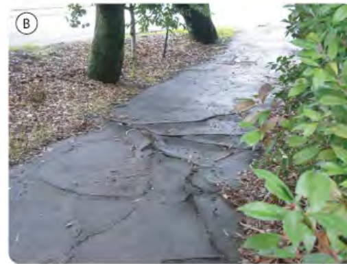
Vineyard south side path: Poor pavement condition
